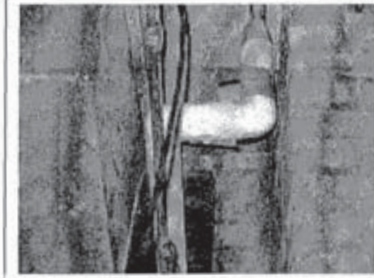
HA - 19: HV-AC Duct Wall & Pipe Insulation
