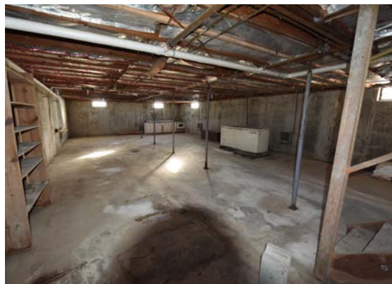
▶ 26' x 408' basement (4) electric wall heaters
