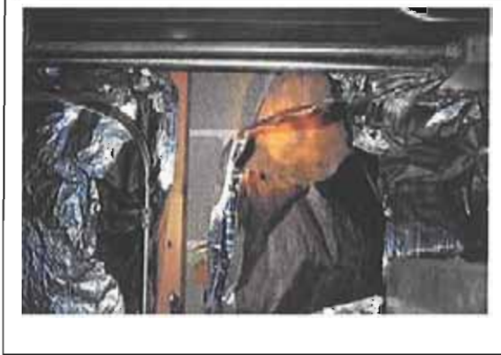
HA - 8: Vapor barrier attached to fiberglass pipe wrap
